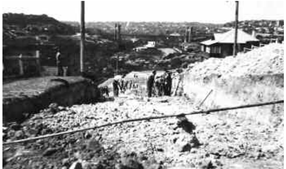
Relief workers during the Great Depression rebuilding Market St in Willoughby in 1935, with Flat Rock Gully and the Suspension Bridge in the distance.
